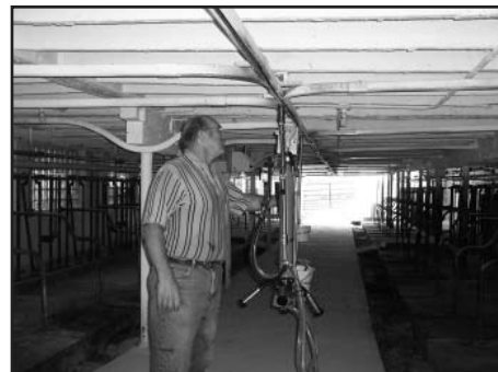
The track system installed throughout the barn allows Schmidt to attach the units with in the milk house and push the units along the track during milking.
