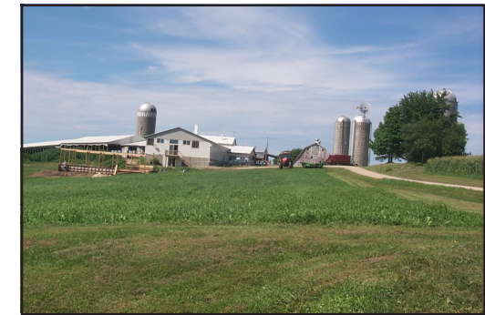
Current calf barn construction among one of the many building projects at Linder Farm.
