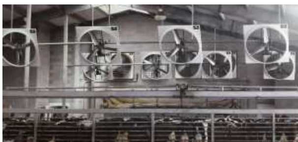
FIG. 9. Circulation fans and sprinklers over holding area.
