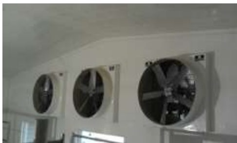
FIG. 8. Positive pressure fans blowing air into milking parlor.
